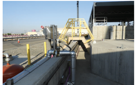
Inland Empire Utility Agency, New Chlorine Injection Facility
