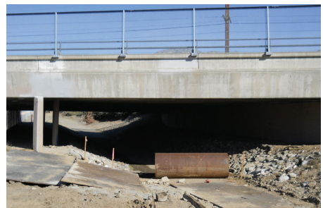
Inland Empire Utility Agency, Recycled Water Pipeline Segment at C-Pipe Supports
