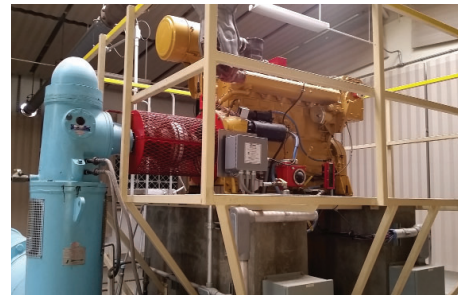
Eastern Municipal Water District Diamond III Booster Plant Pump Electrification, Perris, CA
