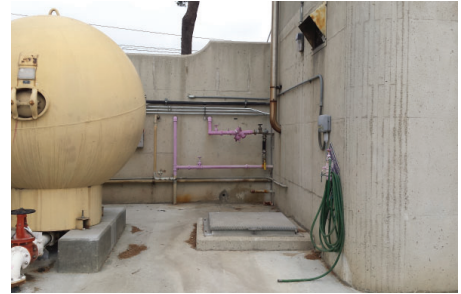
Inland Empire Utility Agency, Pump Station Redundant PLC
