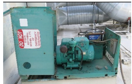
Orange County Public Works Emergency Generators Replacement, Manchester Building - Orange, CA
